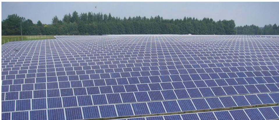
Figure 2. Fixed PV solar plant
