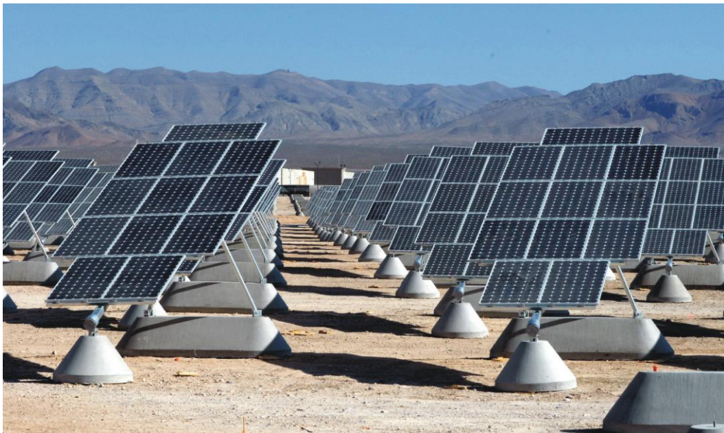
Figure 3. One-axis tracking solar power plant
